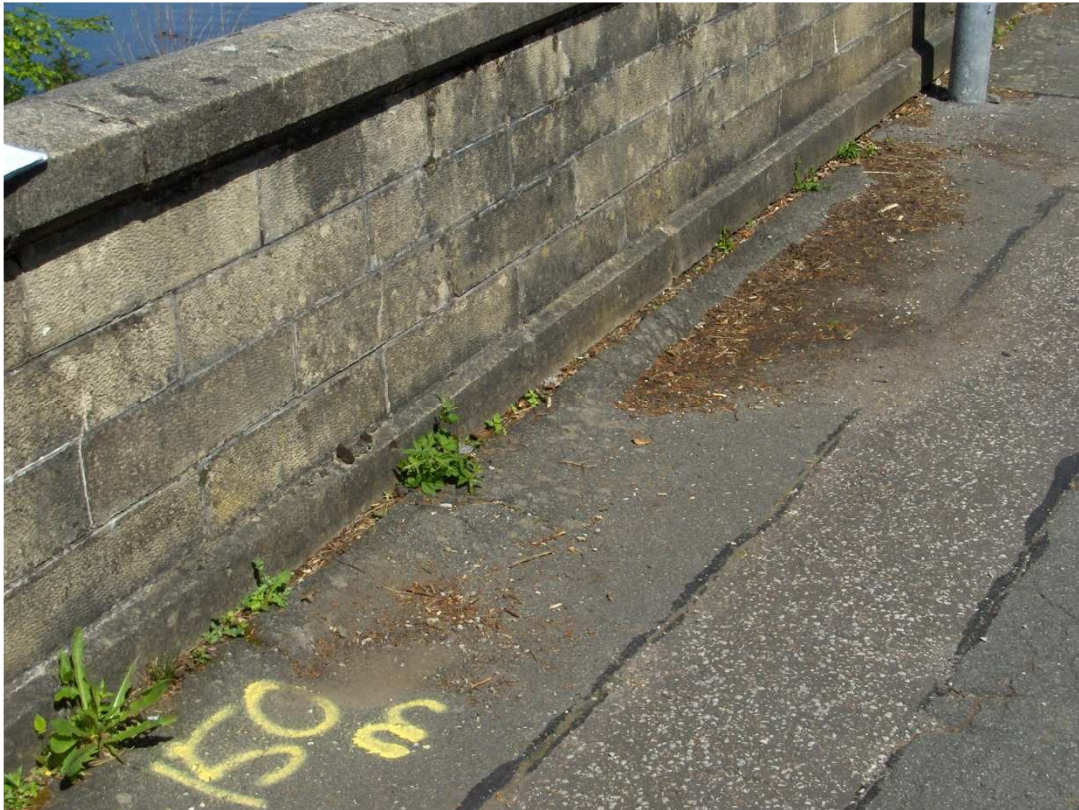
South wall, Chainage 150: Settlement in footpath
