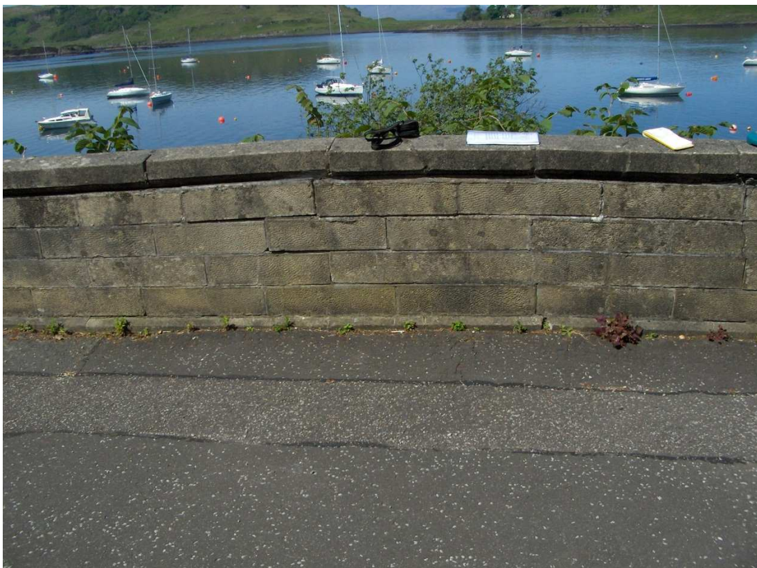
South wall, Chainage 158: Distortion of parapet, probably due to tree growth
