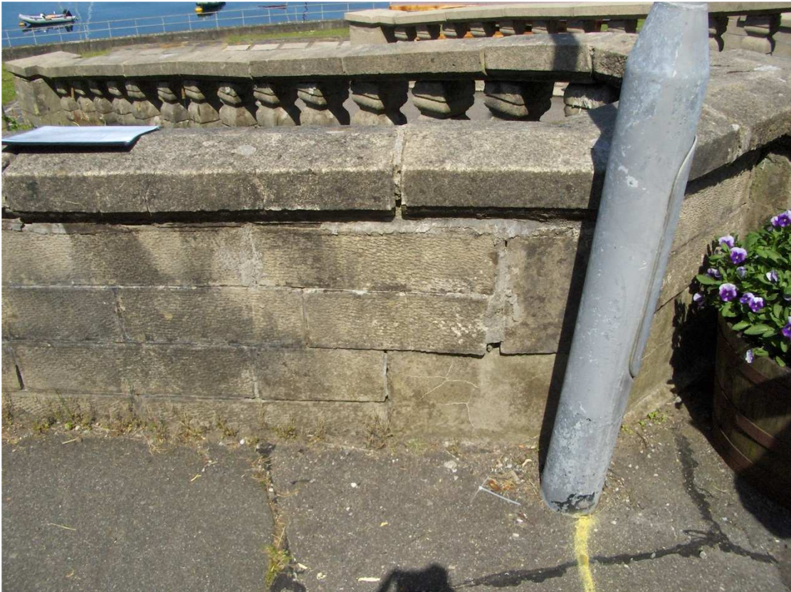
South wall, Chainage 0: Displaced parapet blocks
