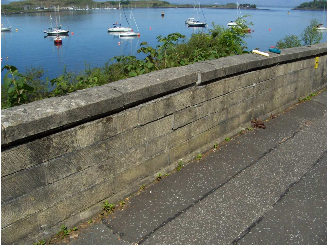
South wall, Chainage 158: Distortion of parapet, displaced cope
