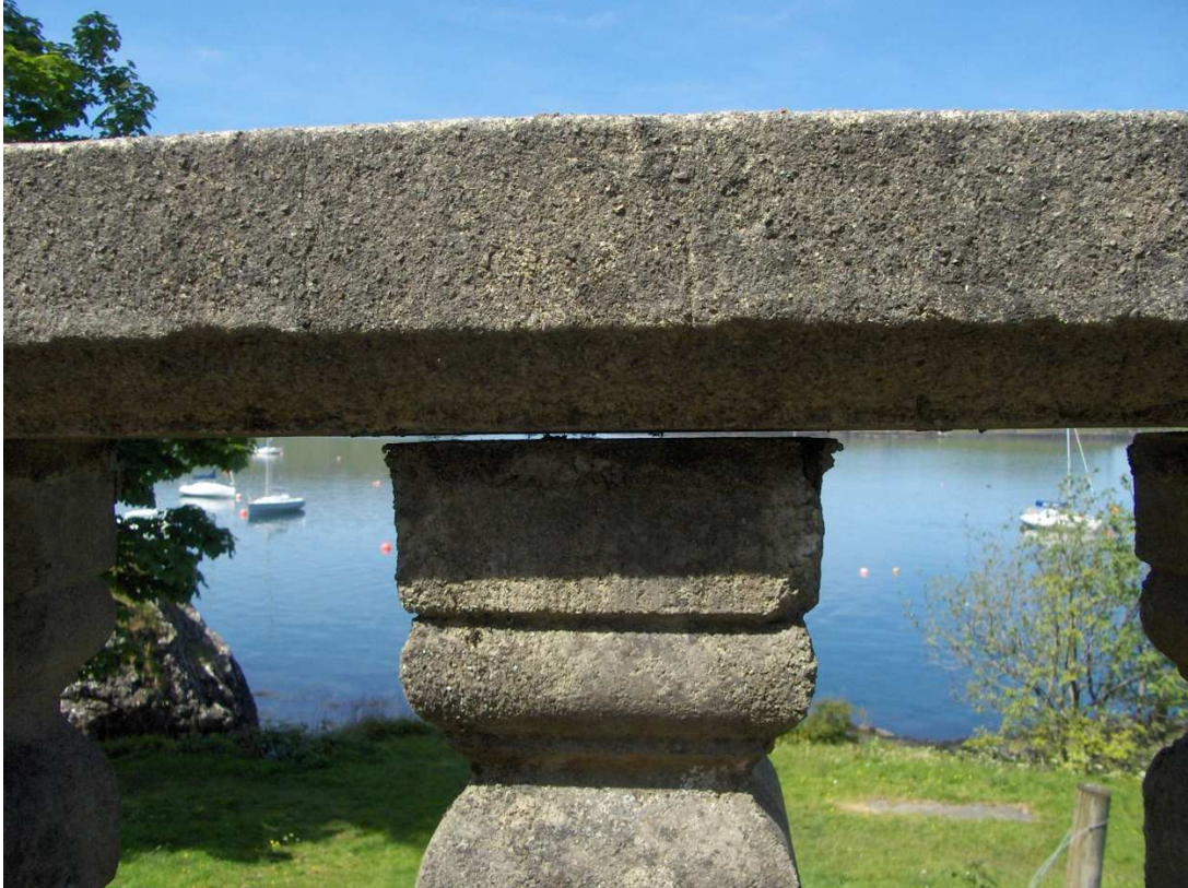
South wall: Loose pilaster (typical)
