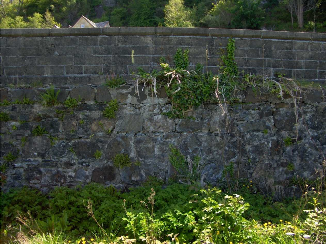
South wall: Ivy growth at Chainage 150
