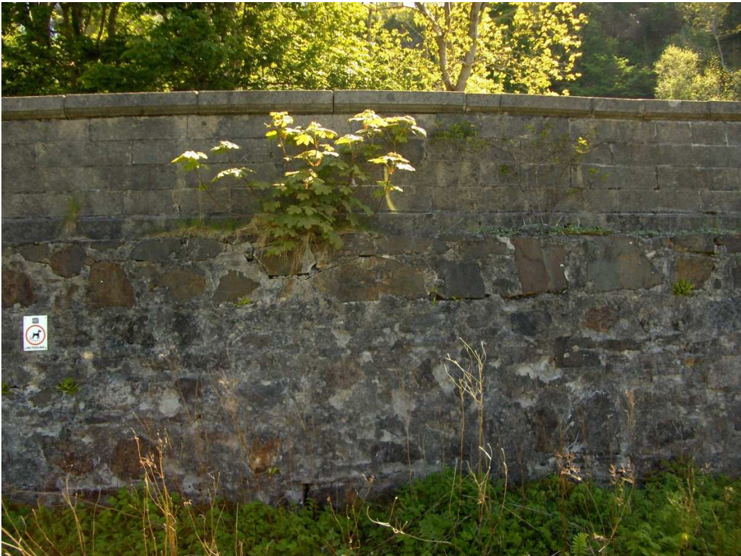
South wall, Chainage 120: Tree growth
