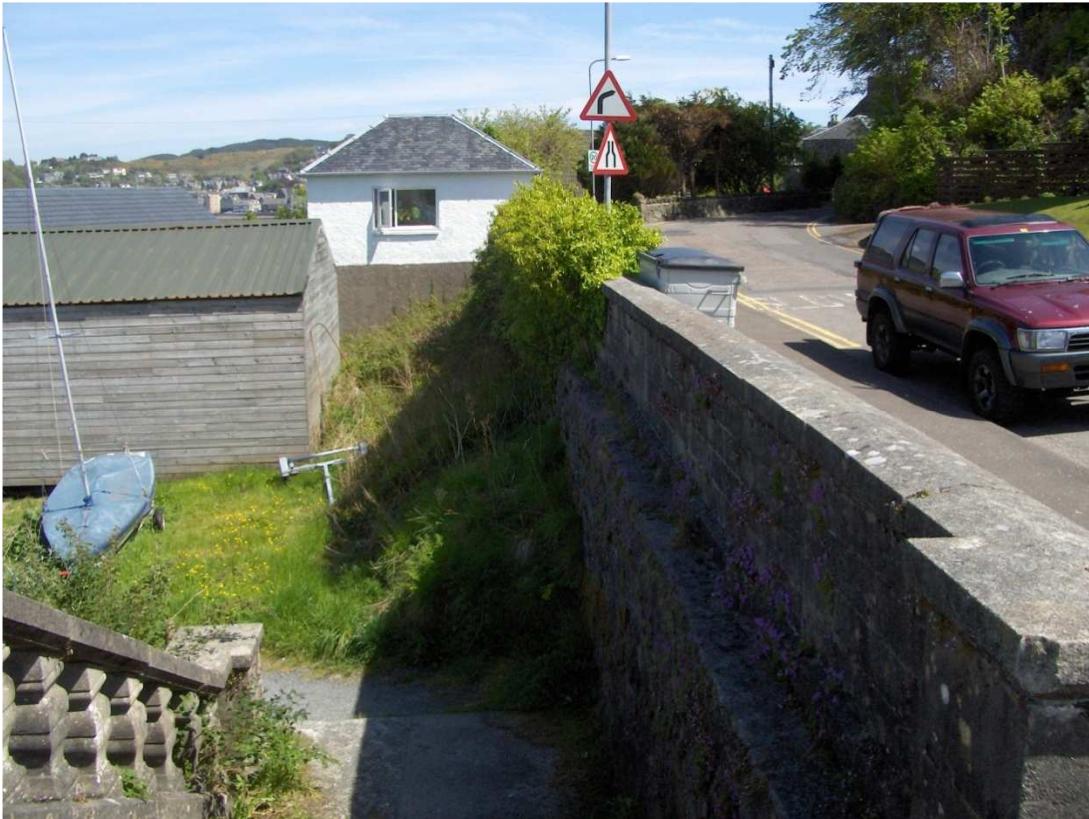
North wall, Town centre end: Dense ivy growth
