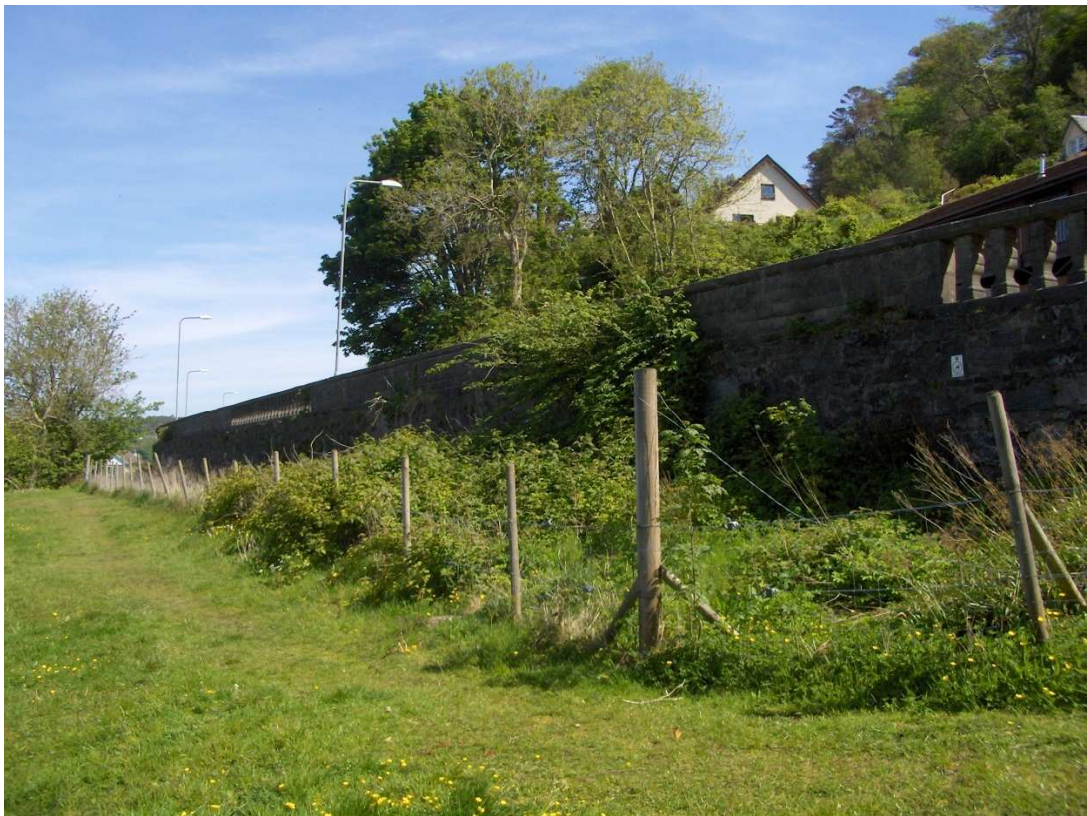
South wall: Tree growth at Chainage 158
