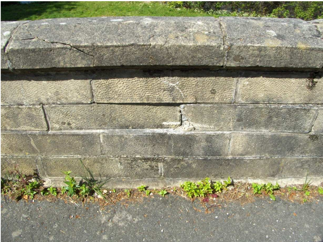
South wall, Chainage 163: Impact damage
